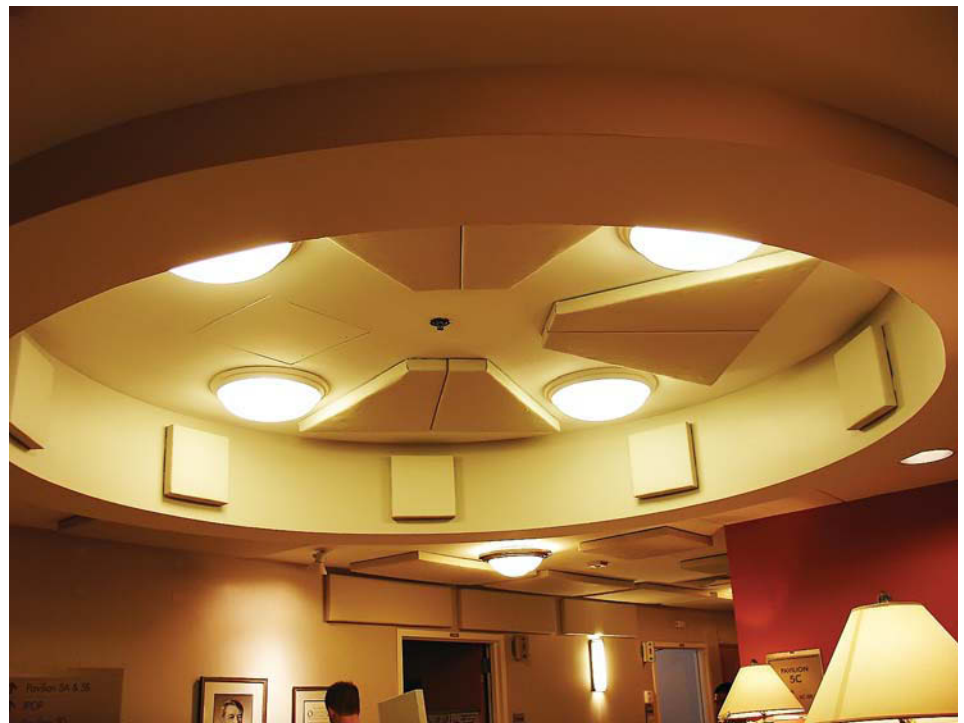
Fig. 3. View of the acoustically absorptive treatment in the remodel of a hematological cancer unit. Sound absorbing panels are mounted high on the walls and on the ceiling of the corridor, as well as in the large circular architectural feature at the nurses' station. Note a person shown at the bottom center for scale (Reprinted with permission from ref. 30. Copyright 2007, Acoustical Society of America).
