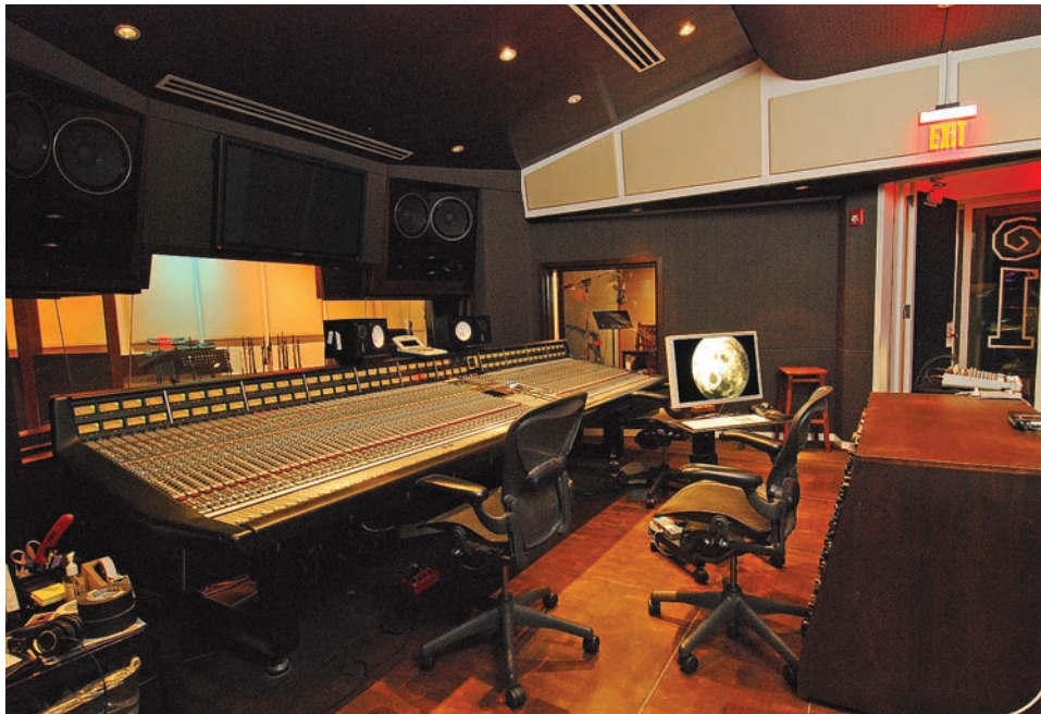
Fig. 1. Interscope Records control room, showing flush-mounted loudspeakers, sloping ceiling, and side soffits.
