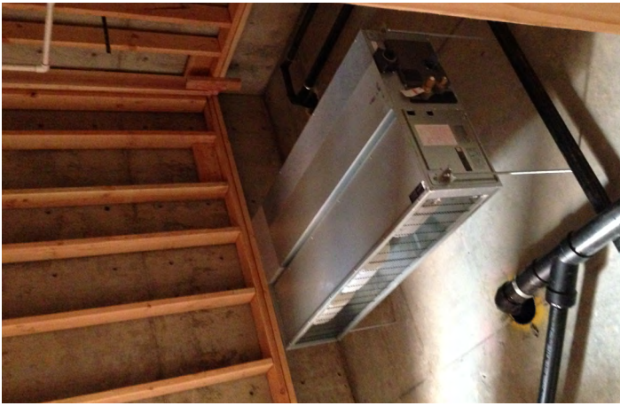
Figure 5. Picture of a loud mechanical unit near a pipe penetration in the ceiling. This figure shows another example of how sounds from a mechanical unit can easily pass through a hole a pipe passes through that has not been acoustically sealed.
