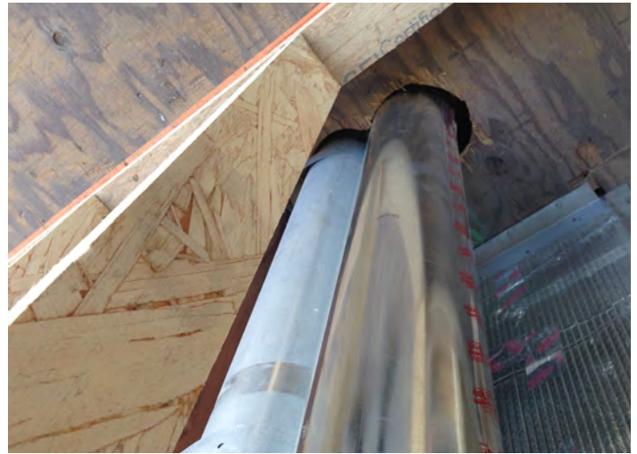
Figure 4. Picture of pipes passing through the floor creating a hole in the floor configuration. This figure shows a typical example of a small hole that degrades the FSTC of a floor, allowing sound to freely pass from one floor to another.
