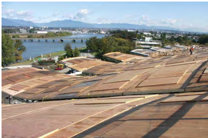
Fig. 2. Curved rooftop under construction with view of the Fraser River and Coast Mountains (Photo by Ziggy Welsch, George Third & Son Ltd., ziggy@third.com Courtesy Wood WORKS! BC).
