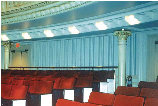
Fig 3. Schroeder diffusers (QRDs ® ) applied to the rear wall of Carnegie Hall to prevent echoes. (After D’Antonio and Cox 17 )
