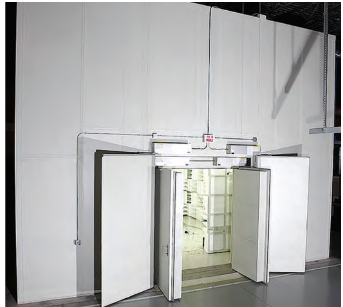
Fig. 8. Completed chamber with double doors open.
