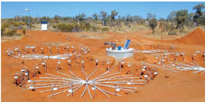
Fig. 2. Partially installed infrasound site in Warramunga, Australia. The pipe rosette will be buried so that only the intakes (white “shower heads”) will be above ground and the four rosettes will be connected to the microbarometer located in the cement vault. (Photo by D. Christie).
