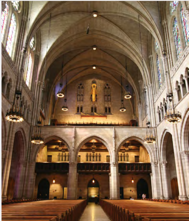
Figure 4. The vaulted ceiling surfaces at the Riverside Church in New York City are Guastavino tile that required sealing after sound reinforcement was added to the sanctuary.
