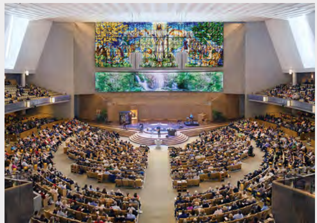
Figure 5. Steerable arrays in the ceiling permit a minimal suspended speaker array system at the Church of the Resurrection in Leawood, Kansas, to serve a large congregation, aiming sound toward the absorptive seating areas and away from the reflective surfaces.
