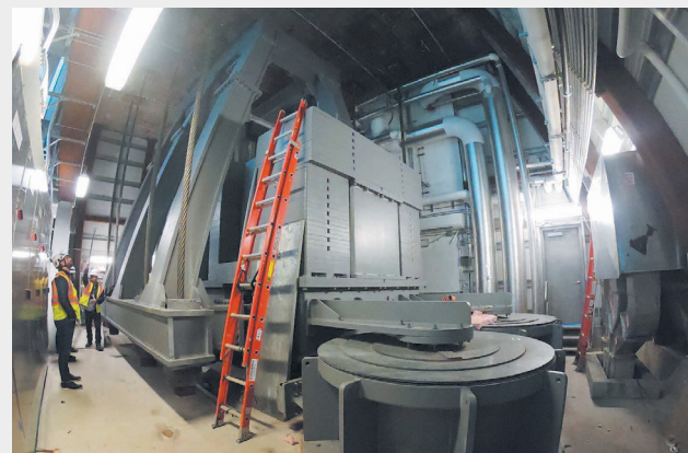
Figure 2. Photograph of a tuned mass damper installed in a tall slender skyscraper. Courtesy of Victor Salcedo of Gerb USA.
