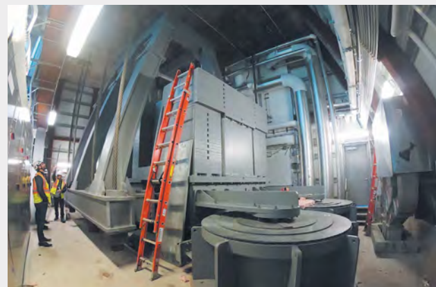
Figure 2. Photograph of a tuned mass damper installed in a tall slender skyscraper. Courtesy of Victor Salcedo of Gerb USA.
