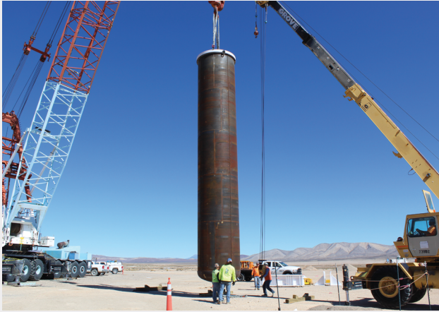
Figure 5. Workers at the Nevada National Security Site (NNSS) emplacing the DAG-2 explosive during the Source Physics Experiment (SPE). DAG-2 was a 50-ton equivalent TNT explosion at a depth of 385 m below the ground surface. Photo from US Department of Energy, taken by a representative of the Nevada National Security Site.
